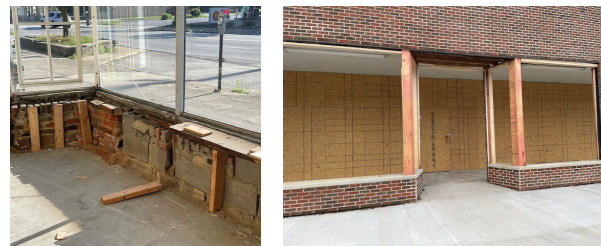
Once completed, the front façade of the building, will offer a clean, refreshed look on Taylor Road.
